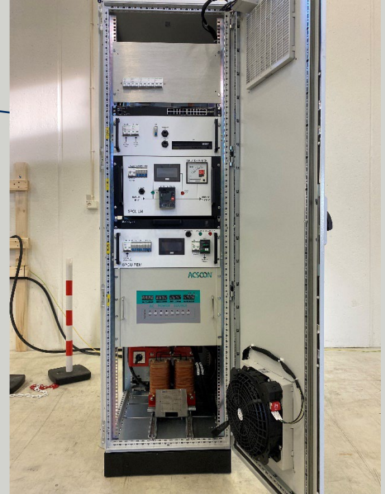
Topside Cabinet (SCU)
