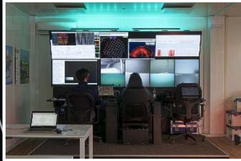
REMOTE/DEPLOYABLE CONTROL ROOM
