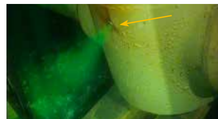
Leakage as discovered October 2012.
