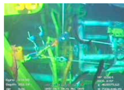
Pull-in arrangement handling a 2nd end flexible towards the porch.
