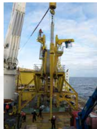
Dynamic end termination deployment
