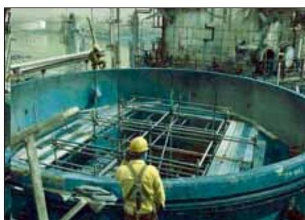
Photo 5 Cracker cut surface
