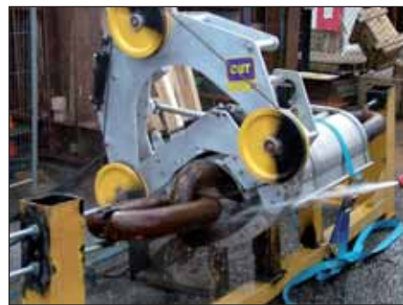
Photo 6 Chain link cutting
