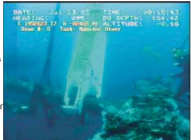
Fig1: Stolt Offshore's 'Parrot Beak' shears being used on the decommissioning of the Eugene Island jacket GOM.
