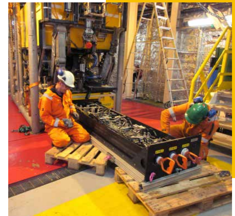
Powerskid installed on the ROV in preparation for the first offshore operation
