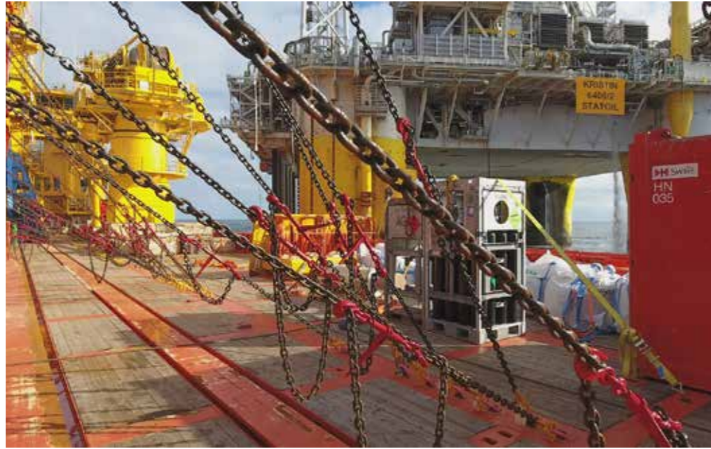
Nice and tidy deck with 5 reels between integrated RDS skidding beams
