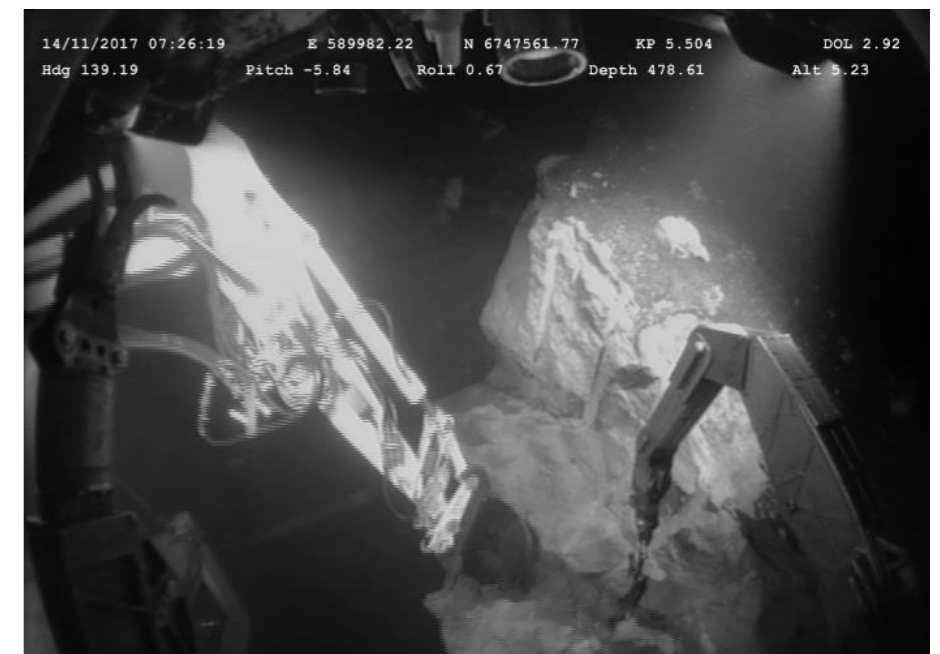
At a water depth of 478 meters, Scanmachine is breaking out a hill side after drilling and use of rock splitters, in close cooperation with ROV.
